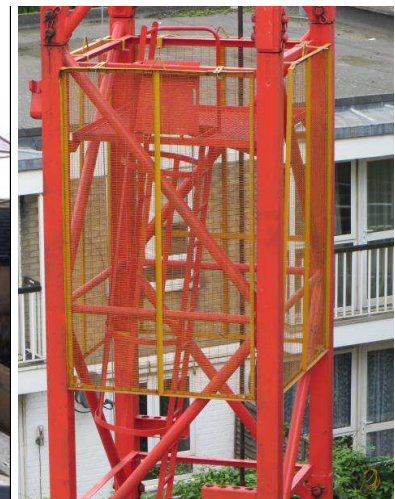
Anti-climb mesh panels
