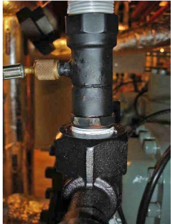
Refrigerant Recovery & Evacuation Point
