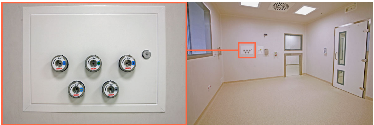
Fig 1 - Gas Outlet Enclosure (5No outlet type Enclosure)
