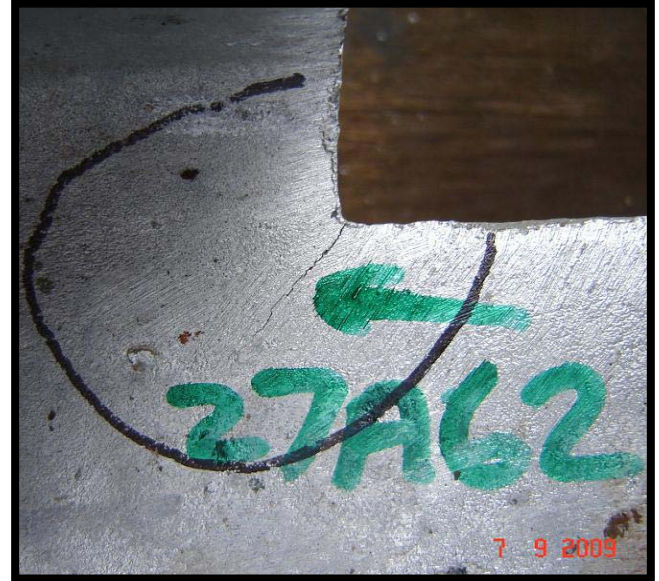
Fig 2 - Bad Notch Detail
