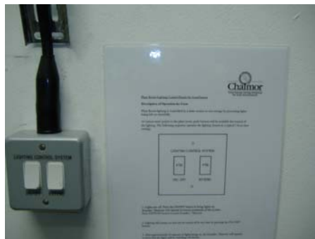
Manual Switch and Signage
