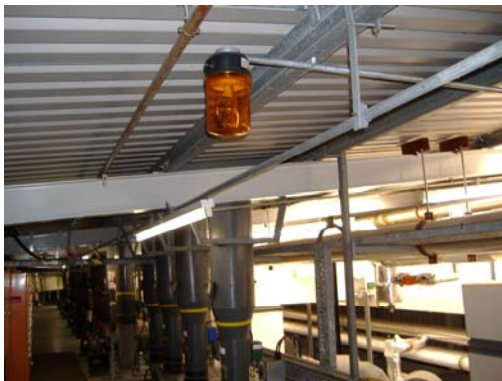
Visible Alarm and a Permanent Egress Light Fitting
