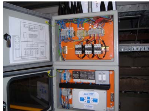
Lighting Control Panel
