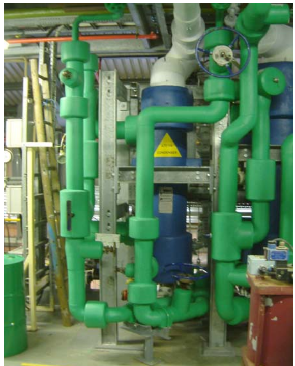
Condenser in final position
