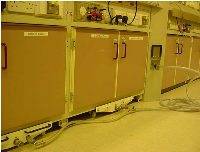
'Hover Pad' trolleys with temporary air connection in readiness for equipment move
